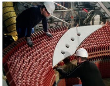
Langenprozelten, Germany 94 MW; HIPASE-E excitation for the world's largest single phase generator
